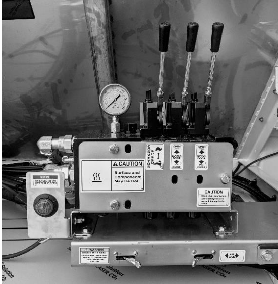
Figure 119- Manifold with wet seal and air lock flipper valves
